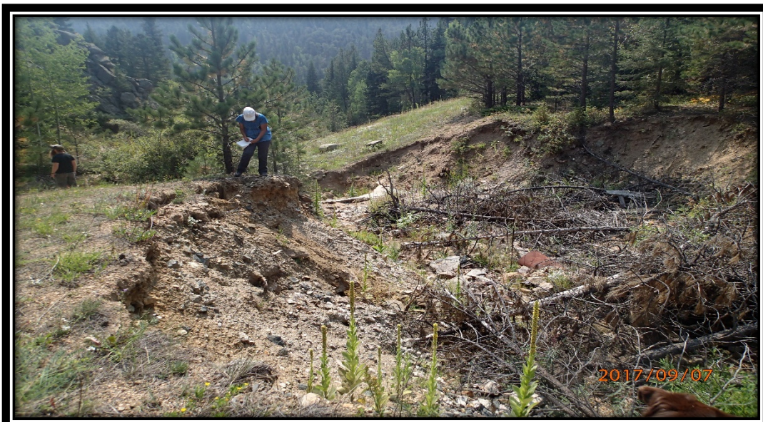
Photos #14, #15 and #16- Cut Bank Slopes and Repository Pre and Post-Reclamation Looking Downstream
