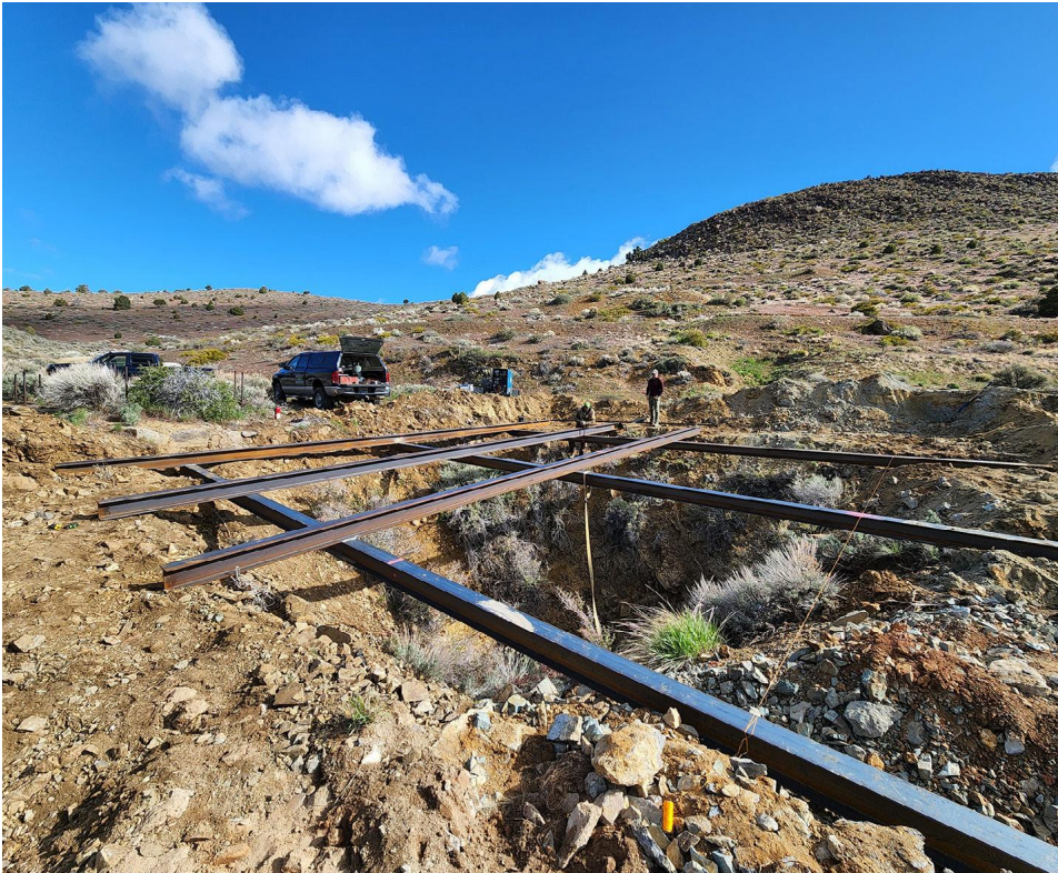
Bat compatible grate built over Sutro Air Shaft #3 with construction techniques used for cultural avoidance.
