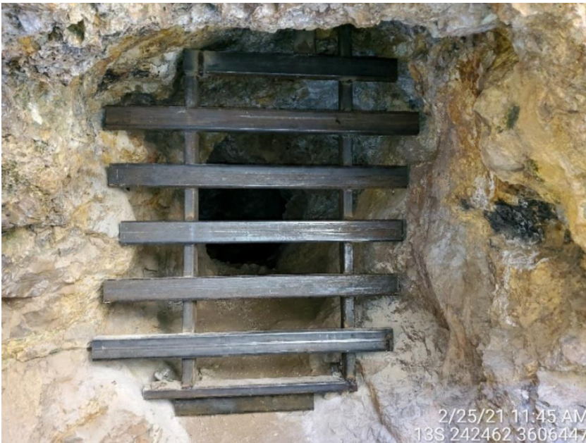
Bat Gate constructed by MineGates Environmental in a very remote location.
