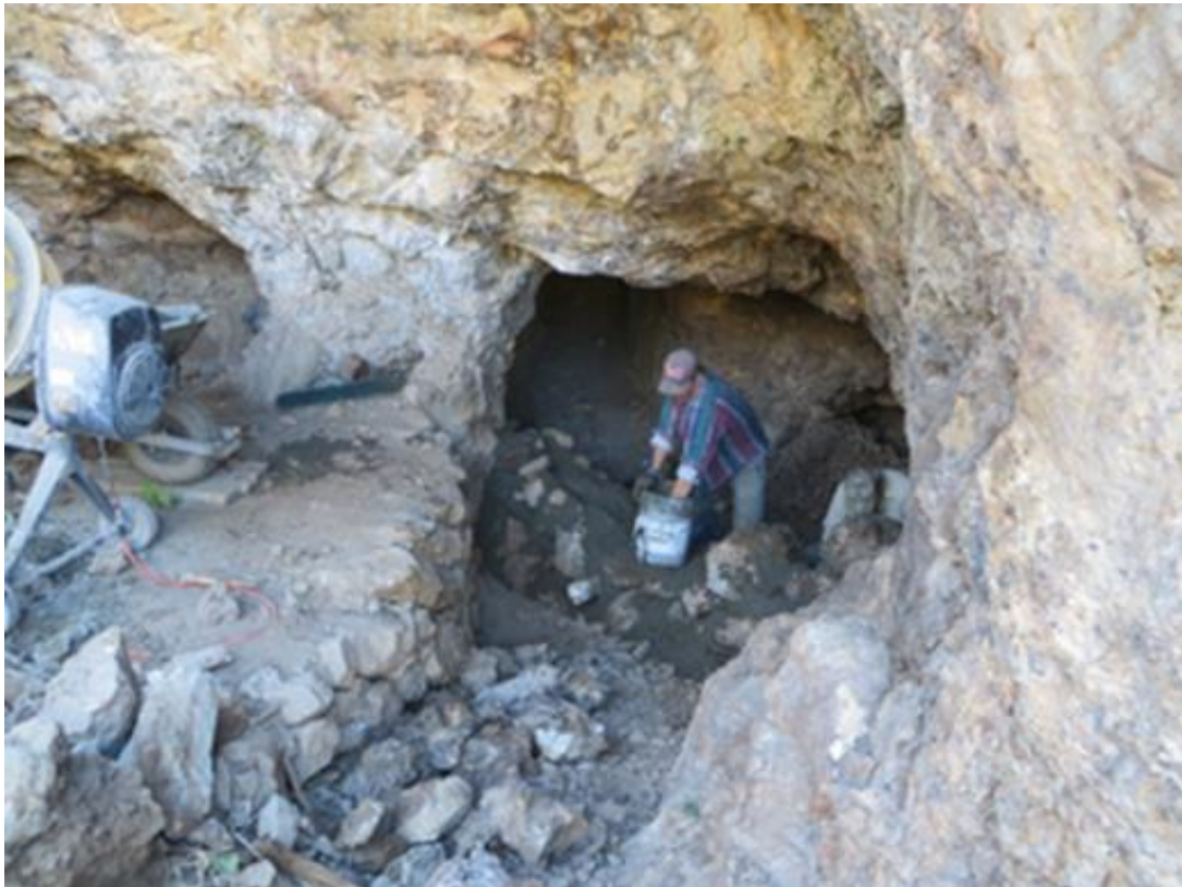
Feature 24 receiving two rock bulkheads with bat gates
